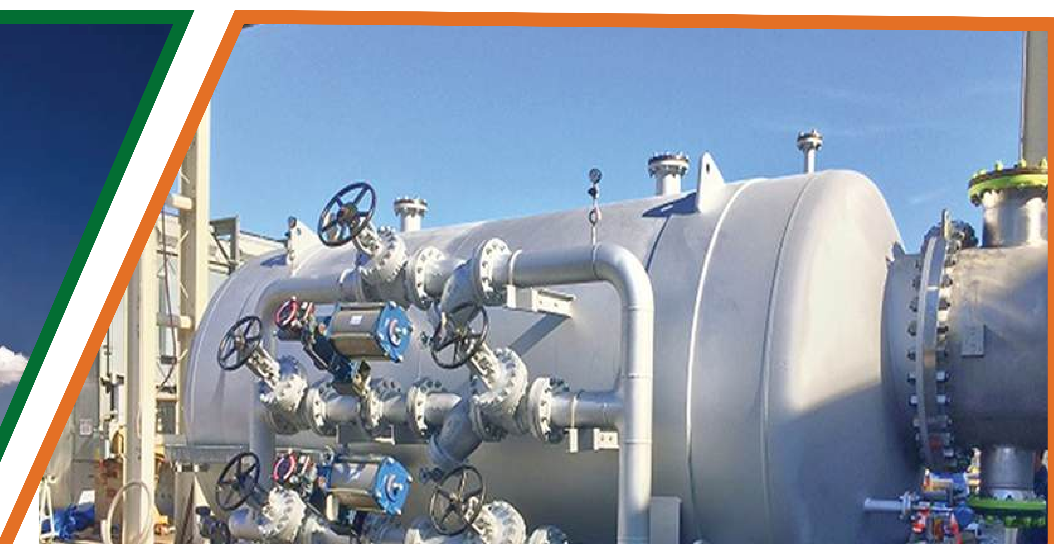
Pressure Vessels & Boilers etc.
