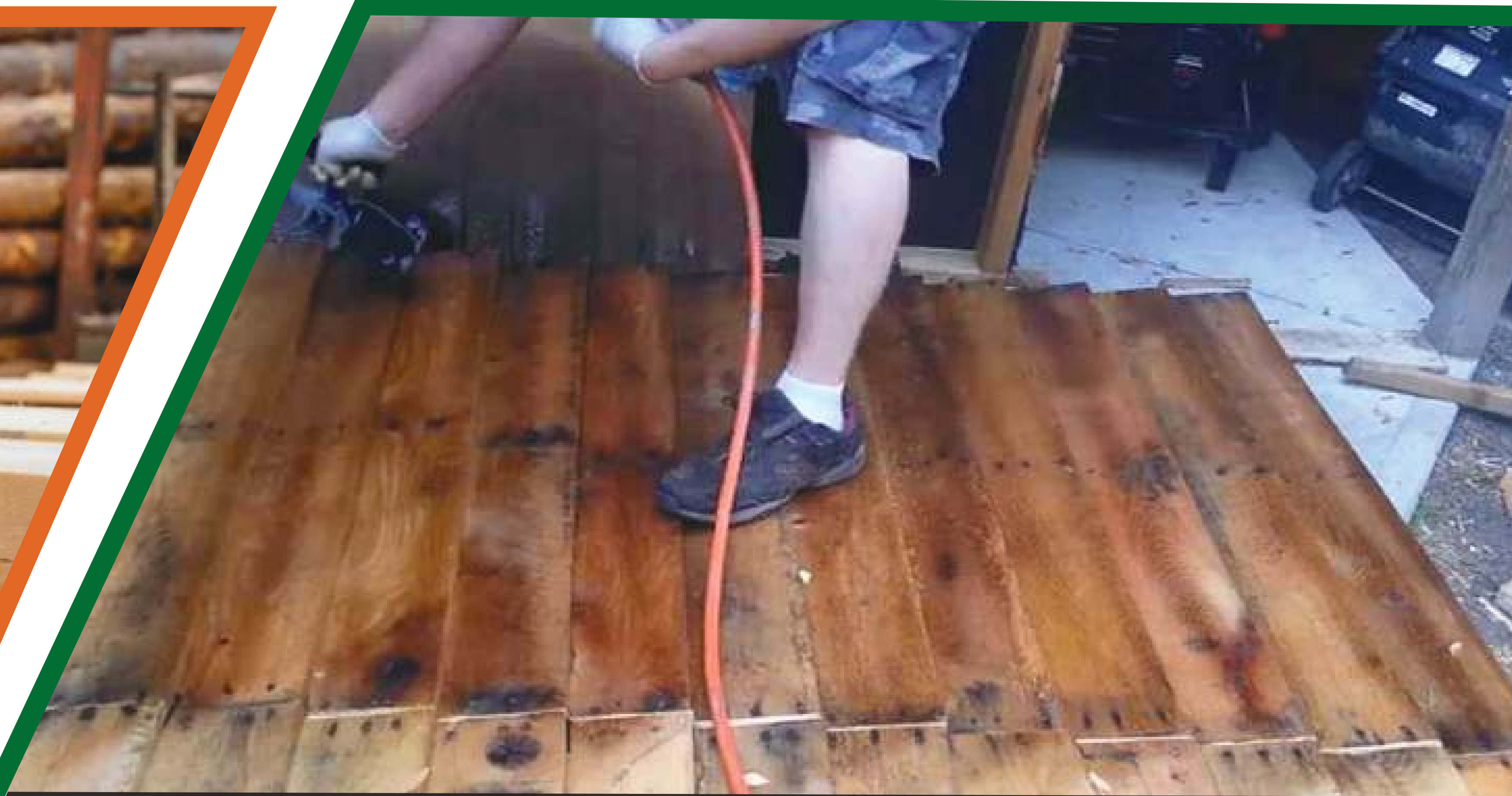
Diesel/Oil Soaked Wood
